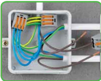
Wiring of flexible conductors in a junction box
